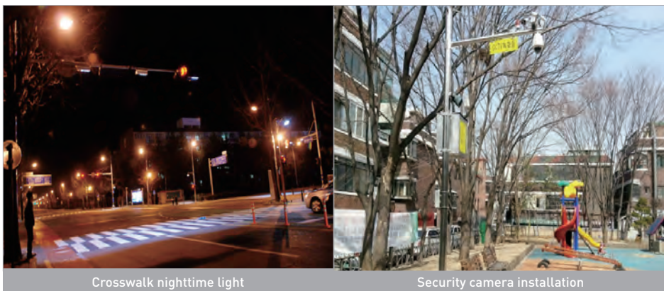
Figure 5.5 Examples of installation and repair of facilities in a zone subject to pedestrian environment improvement
